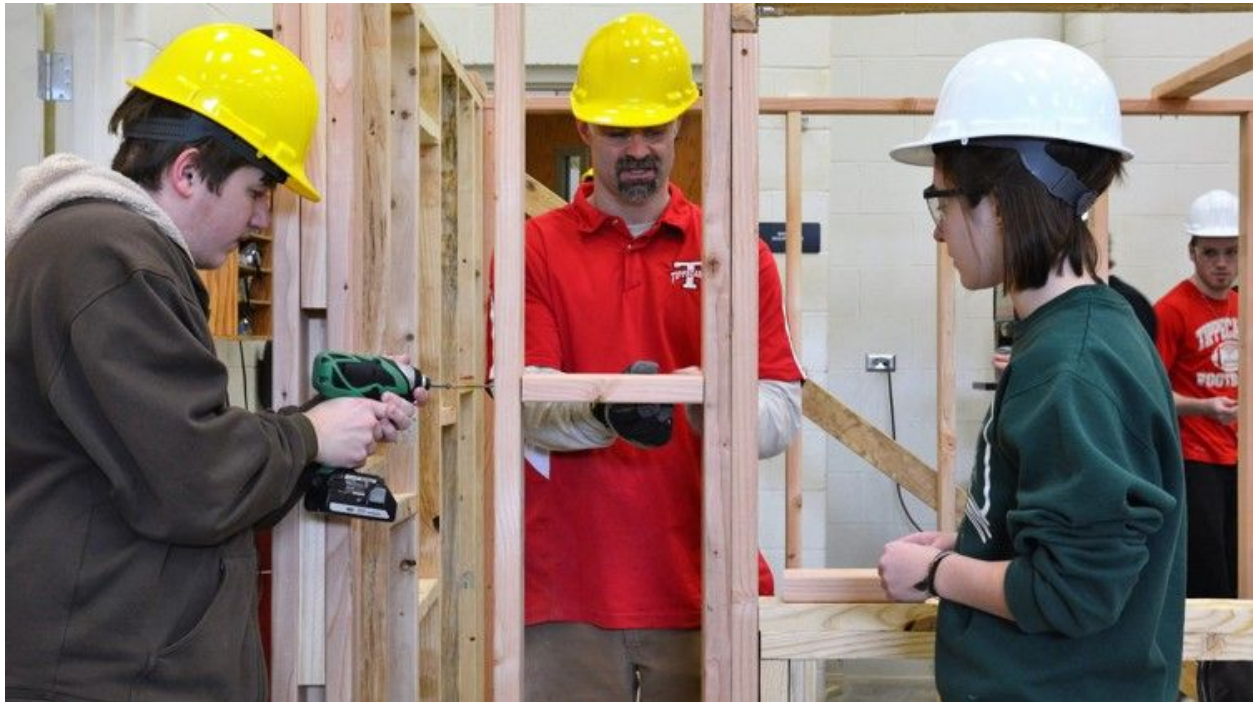
Instructor Jim Kitchen (center) works with Tippecanoe High School students working to build a tiny house. CONTRIBUTED
